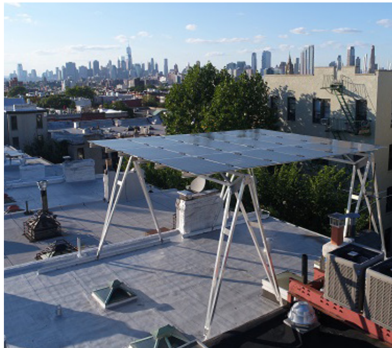
A solar canopy on a building in New York City. Credit: Solar United Neighbors/Brooklyn SolarWorks
