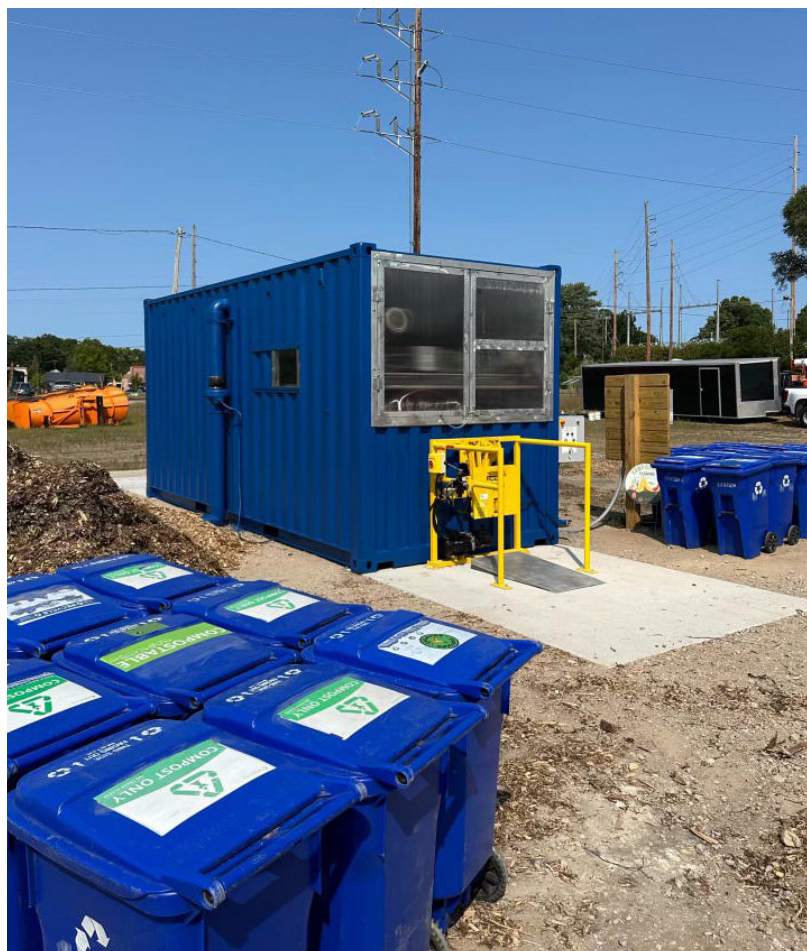
Painted in-vessel compost system in Traverse City, MI Credit: City of Traverse City
