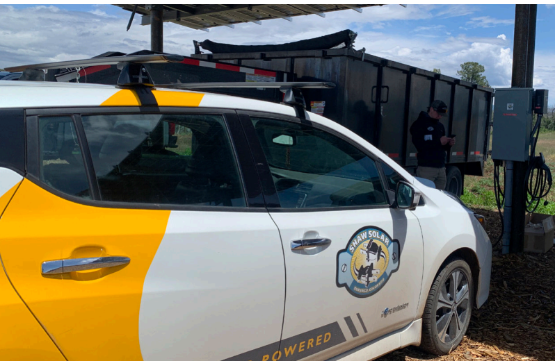
Solar station charging electric vehicles Credit: Table to Farm
