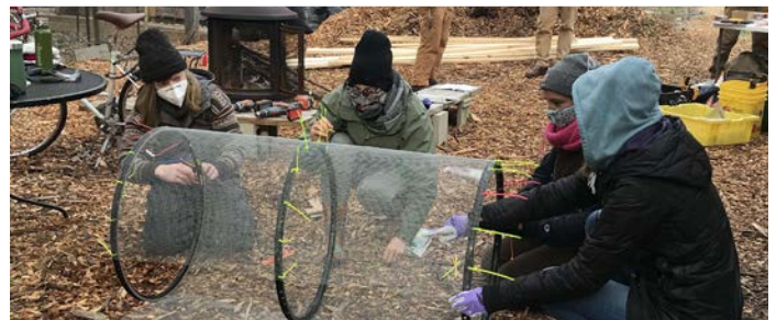
▲ Volunteers build a compost screener made, in part, from repurposed bicycle wheel rims at Hidden Harvest Farm, an event organized by ILSR and sponsored by the Baltimore Office of Sustainability. Photo Credit: Brenda Platt
